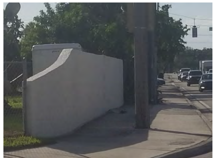
Existing wall at NW 19 St to be replaced
