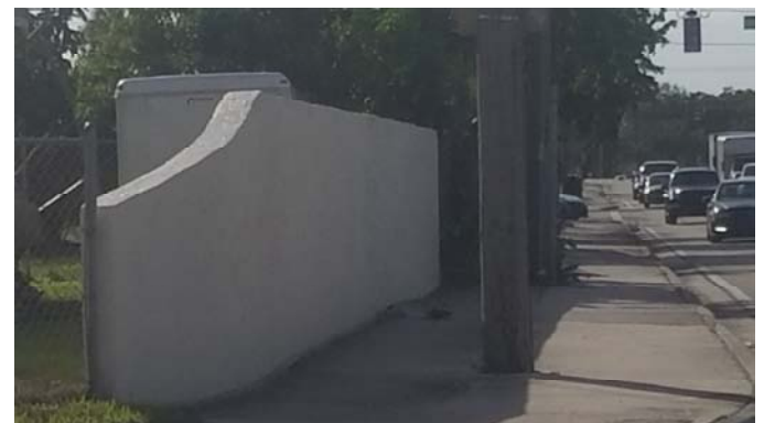
Existing wall at NW 19 St to be replaced at a future date
