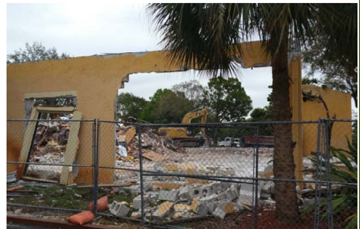
Demolition of the old Annex on NW corner of City Hall site was completed in February
