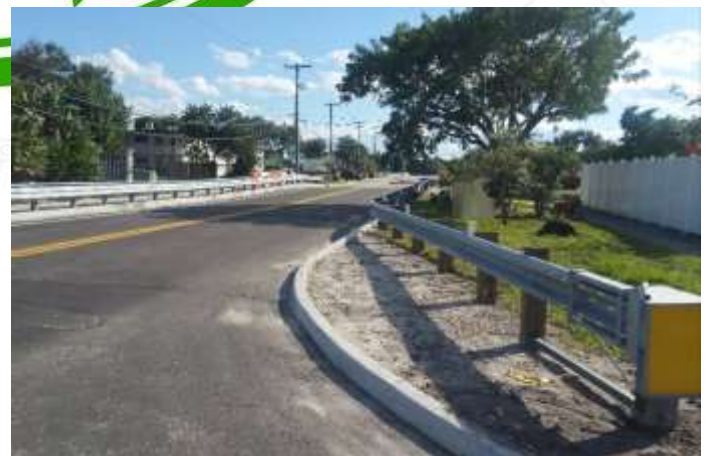
NW 47 Ave has re-opened from NW 26 St south to Sunrise Blvd
