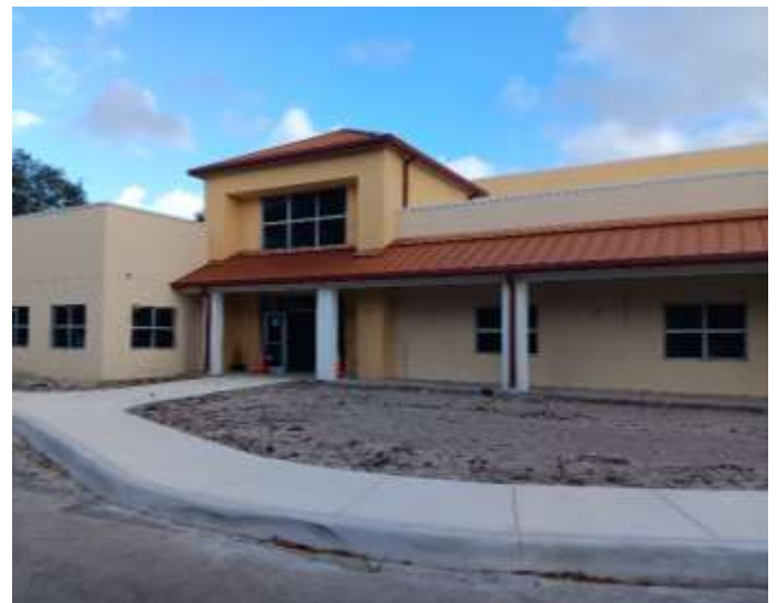
Ahrens Construction has completed the foundation and outside walls and begun interior buildout
