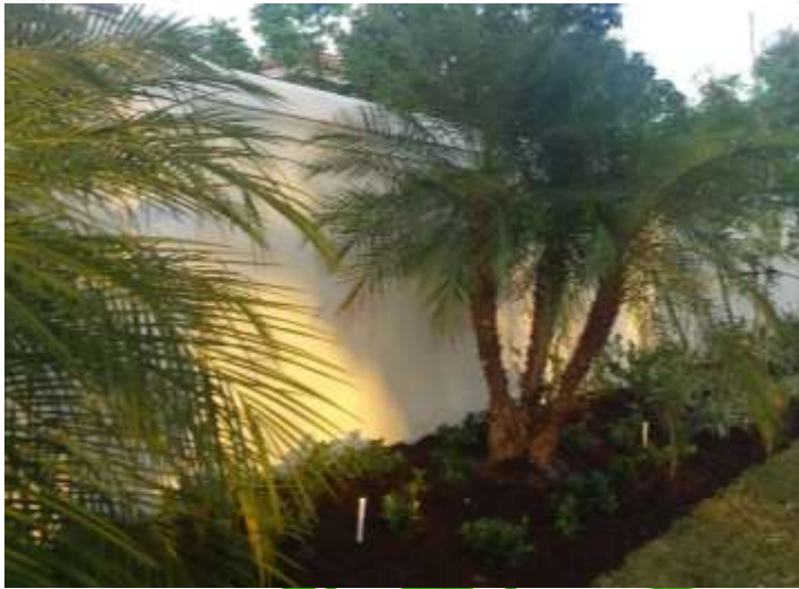
West Construction has completed the landscaping and irrigation installation along the new wall
