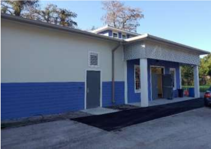
West Construction has completed exterior finishes and is completing interior buildout and painting.
