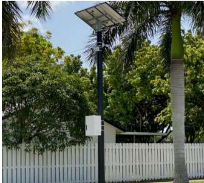
New poles for the cameras and license plate readers can be combined with solar panels for standalone operation
