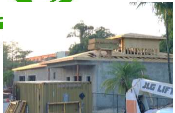
Building under construction showing foundational work prior to paint and finishes (top left picture)
