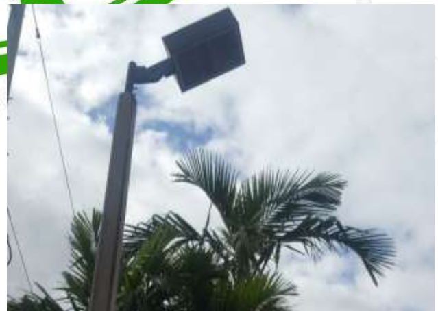
Older lighting replaced in parks was not energy efficient and exceeded light spill standards
