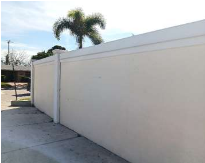
Construction is complete on the new wall along NW 19 Street east of State Road 7
