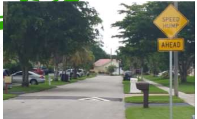
Speed hump installation has been completed at many new locations throughout Lauderhill
