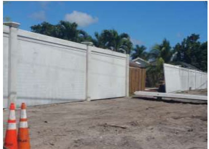
After demolition of the existing wall, the precast posts and panels for the new wall can be installed quickly by lowering into place
