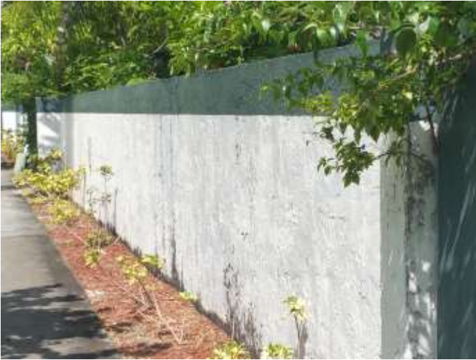
The existing walls on NW 44 St and on Inverrary Blvd did not match City design or standards
