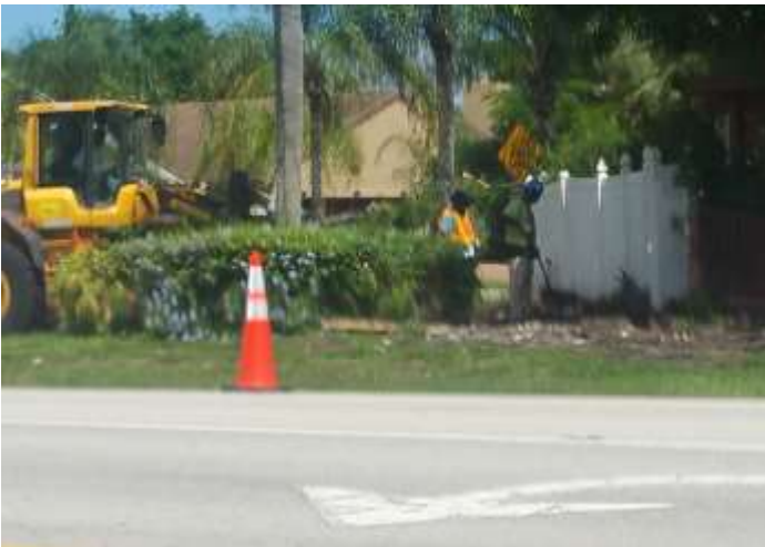
Work crew from MBR Construction removing vegetation and preparing for existing wall demolition
