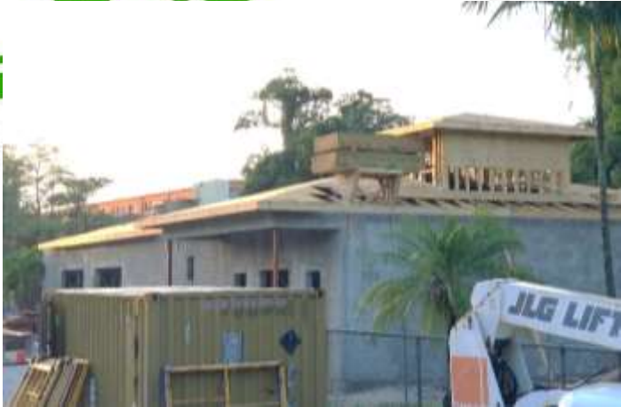
Building under construction showing foundational work prior to paint and finishes (top left picture)
