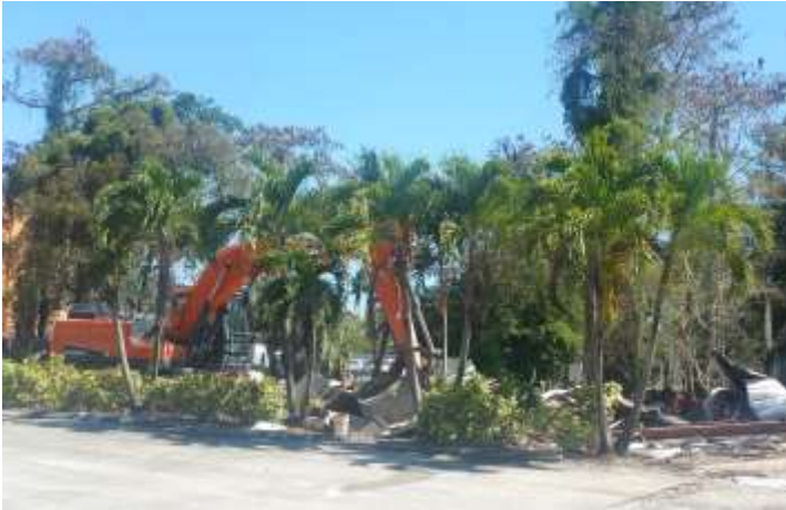
Demolition of the old maintenance metal frame building at the Golf Course
