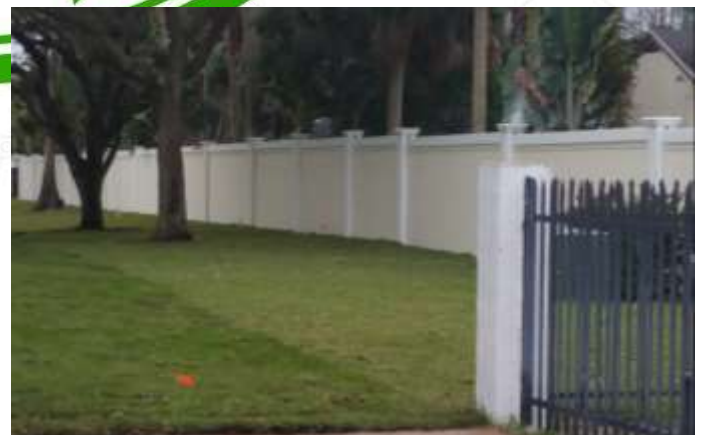
Construction of the new privacy wall has been completed to replace the mismatched fencing on west side of park.
