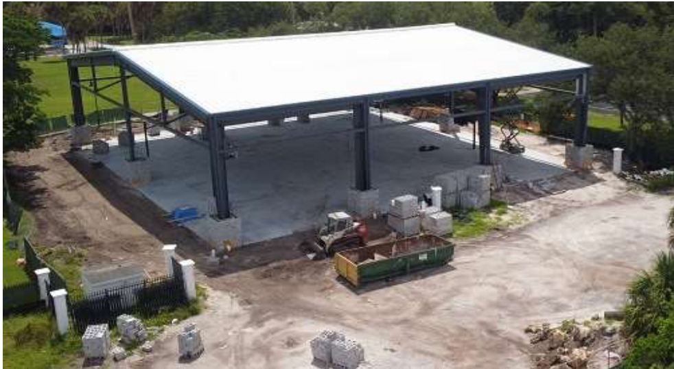
Below: Erection of steel frame and installation of roof for basketball court covers
