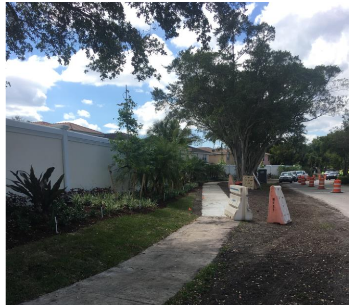
Landscaping and new irrigation was the last step in the installation process
