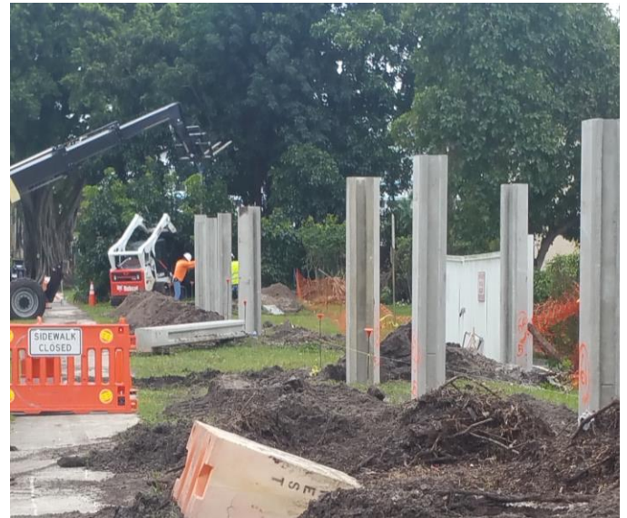
Wall mounting posts were installed prior to the panels being lowered into place
