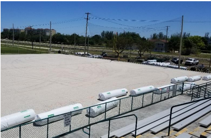
Field turf rolls ready to be laid out by the contractor to complete the installation
