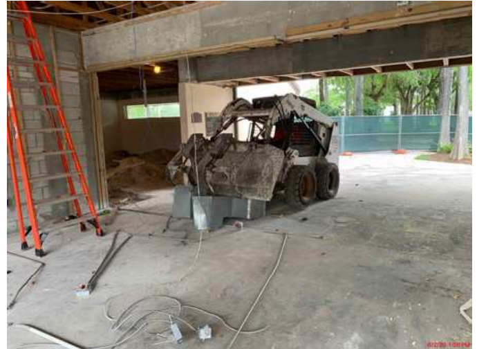
The interior of the building is being completely renovated, including floors and walls
