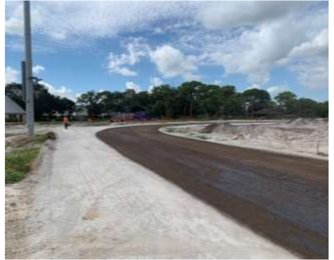
Progress photo of new running track with gravel base and first layer of track surface
