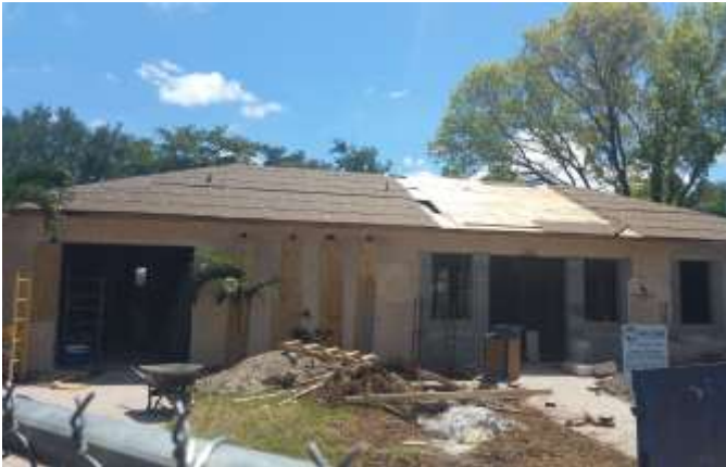
The existing building was closed and interior was stripped out for renovation
