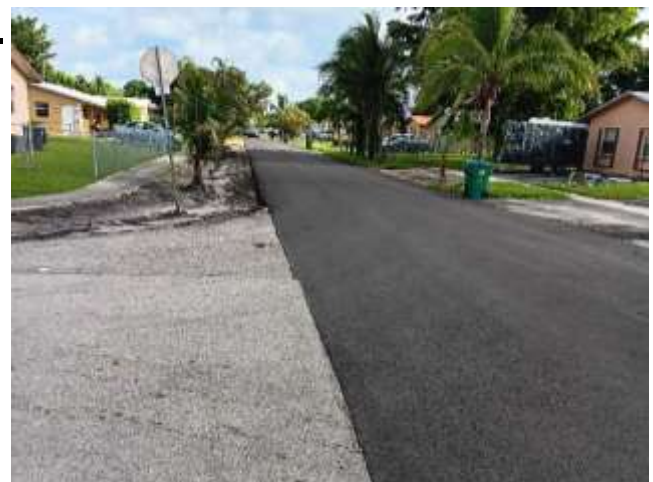
Roadways are resurfaced on a schedule for safety and to reduce repair costs. Area at NW 17 Court shown above.
