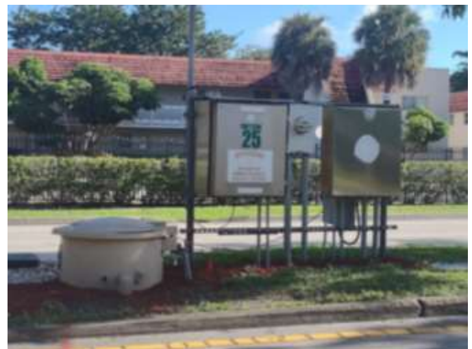
Lift stations and pumps move wastewater from gravity lines connected to homes and businesses
