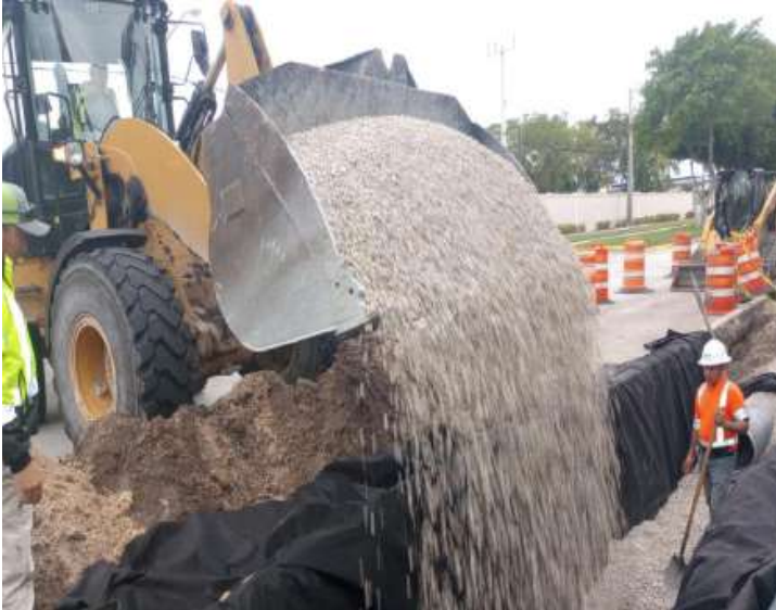
Southern Underground has completed installation of new interconnect with Sunrise water system on NW 44 St
