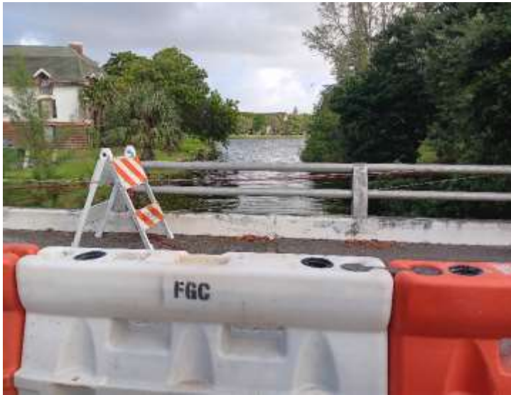
FG Construction has started bridge repair work in Inverrary to include two on Inverrary Blvd and one on Inverrary Drive
