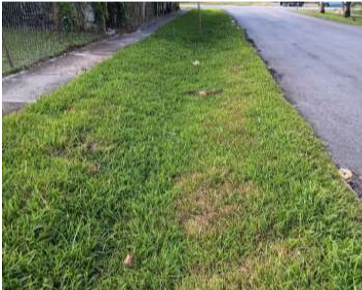
Completed swale on NW 17 Court after work by Weekley Construction to lower and re-sod
