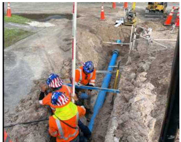
Replacement of water lines on Lime Hill Road has been completed. NW 82 Ave will be the next water line upgrade.
