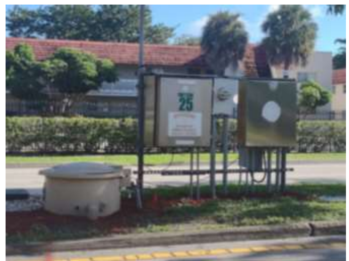
Lift stations and pumps move wastewater from gravity lines connected to homes and businesses
